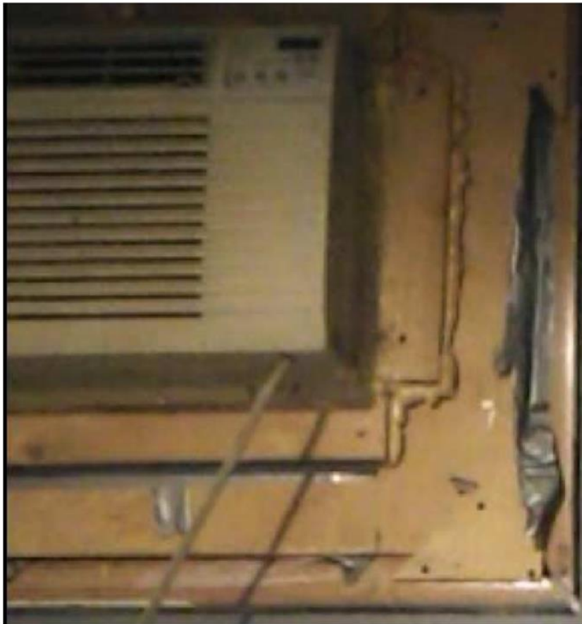
(above) SS001: Air Conditioning Unit
